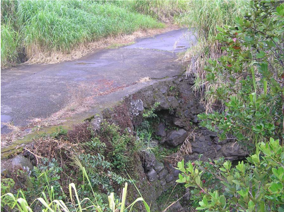
Figure 1. Existing stream crossing at the Kapili Stream. Notice the actively eroding undercut just right of center in the photo.
